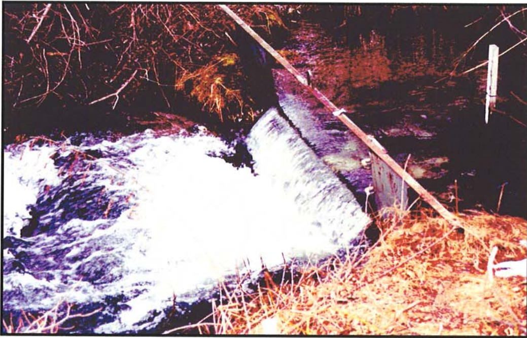
DEP uses this measuring weir to monitor the millions of gallons of leaking Delaware Aqueduct water that rise daily to the surface in Newburgh. Photo by William Wegner.
