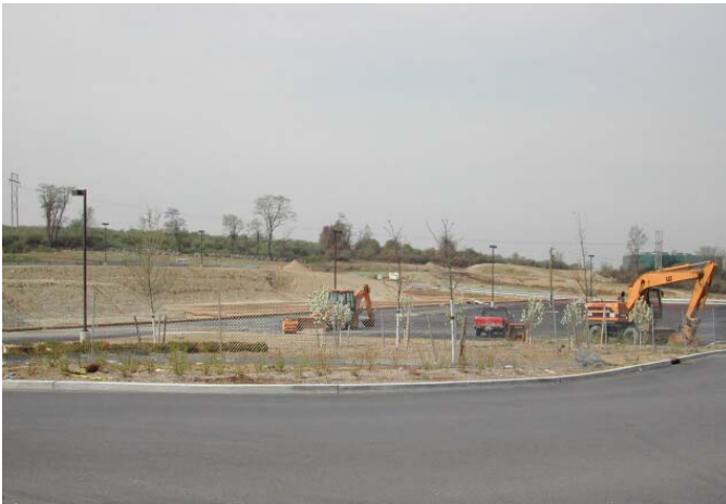
Acres of pavement being constructed to serve big box stores located near Interstate 84. Photo by Marc A. Yaggi
