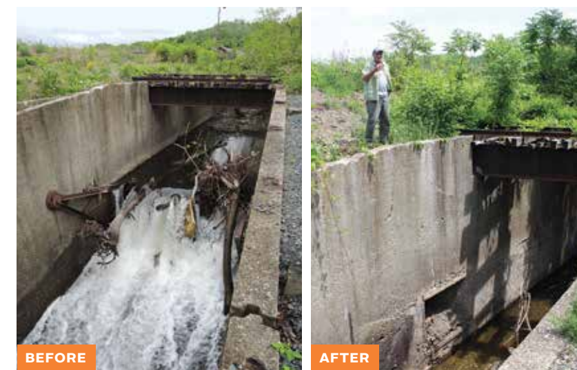
Wynants Kill, before and after the removal of the dam. Frances Dunwell of DEC’s Hudson River Estuary Program said the dam “was like a clogged artery for the river, and the clog is gone.”
