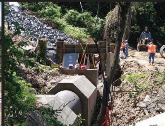
The workers are preparing to install the replacement pipe. Note how steep the slope is – another landslide waiting to happen?
