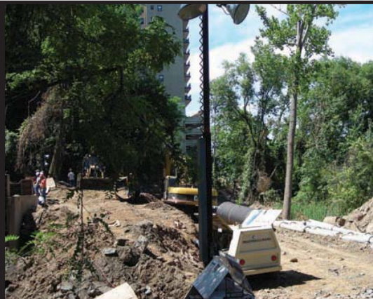
Here is a view of the ongoing work from the hill where the sewage pumps are located, looking towards the Greystone train station and the adjacent residential development complex. A more extensive project is proposed for this location despite the site’s demonstrated instability and the importance of the wetlands that remain.
