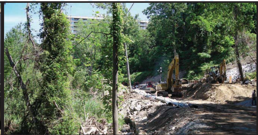
The temporary access road from the Greystone train station side. The remaining wetlands are on the left, and the broken pipe is at the bottom of the steep hill to the right.
