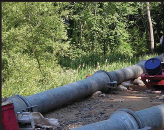
The wetlands that caught, slowed, and absorbed large amounts of the sewage spewing from the ruptured pipe lie beyond the pipes that bypassed the break.
