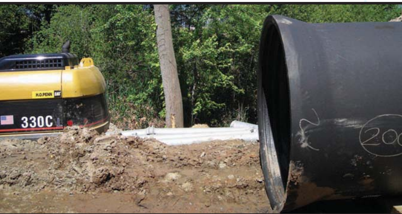
The 48" replacement pipe is in the foreground. Beyond it are the bypass pipes on the temporary fill, the wetland, and the Hudson in the distance.
