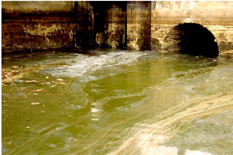
Overflow pipes like this one on Newtown Creek discharge raw sewage and dirty stormwater into New York Harbor and the Hudson River. Image: Giles Ashford © 2004.
