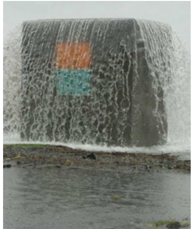
Orangetown and South Rockland sewer districts pipe overflowing during rain
