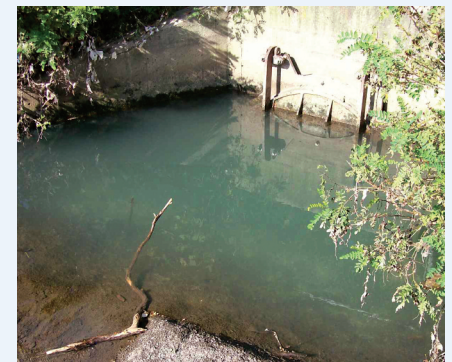
Cloudy water and visible pieces of toilet paper hanging from the scrubs, alerted a citizen to this sewage overflow.
