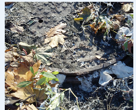
Toilet paper, or other floatables, emerging from a sewer manhole are a sign that sewage has recently overflowed.
