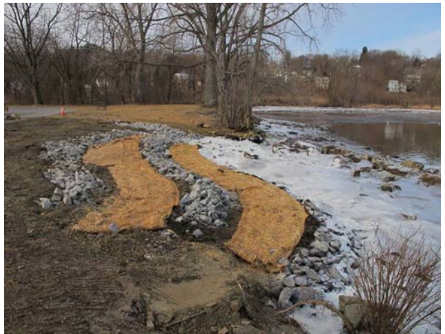
An “ecologically enhanced, engineered shoreline” was built in Cossack, NY. The shore included a series of terraces made of stone and plantings. The shoreline was designed to protect a public parking lot while enhancing shoreline and river habitats.
