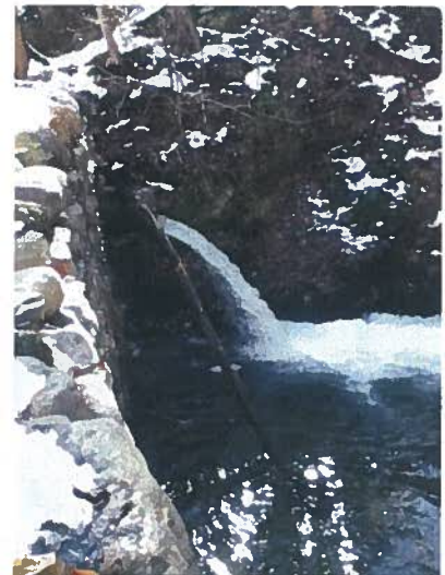
Figure 3. A greater than 30 foot tall dam located at the end of Segment 1 of Hunns Lake Creek.
