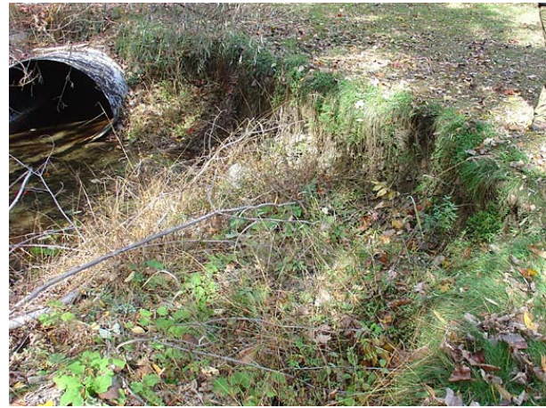
Culvert with Erosion 18.
