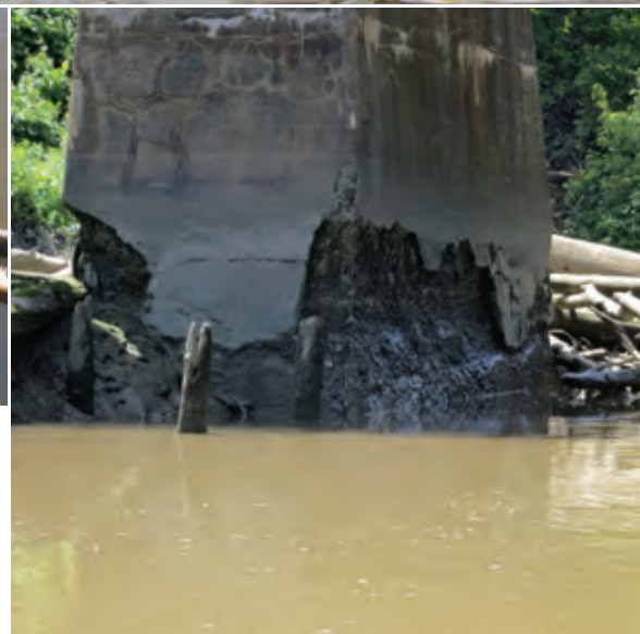
6/17/2015: Another crude oil rail bridge rotting to hell. This one over the Normanskill near Albany. Our initiative on crumbling rail bridges led to a nationwide effort by Waterkeepers all across the country who documented deteriorating bridges for a report to federal agencies and elected officials. Will our government, so focused externally on national security, have the integrity to address this real and imminent risk?
