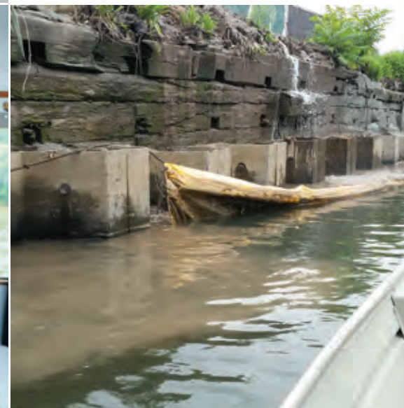
7/2/2015: We found this turbid discharge from a construction site during our Gowanus Canal patrol. We reported it in real time to DEC, our community partners and the press. Within a couple hours the developer had heard from all three, DEC did well and issued a violation. Message to developers hoping to capitalize on the anticipated Gowanus cleanup... "Make very sure you don't cause the slightest harm to the waterway and its aquatic life."
