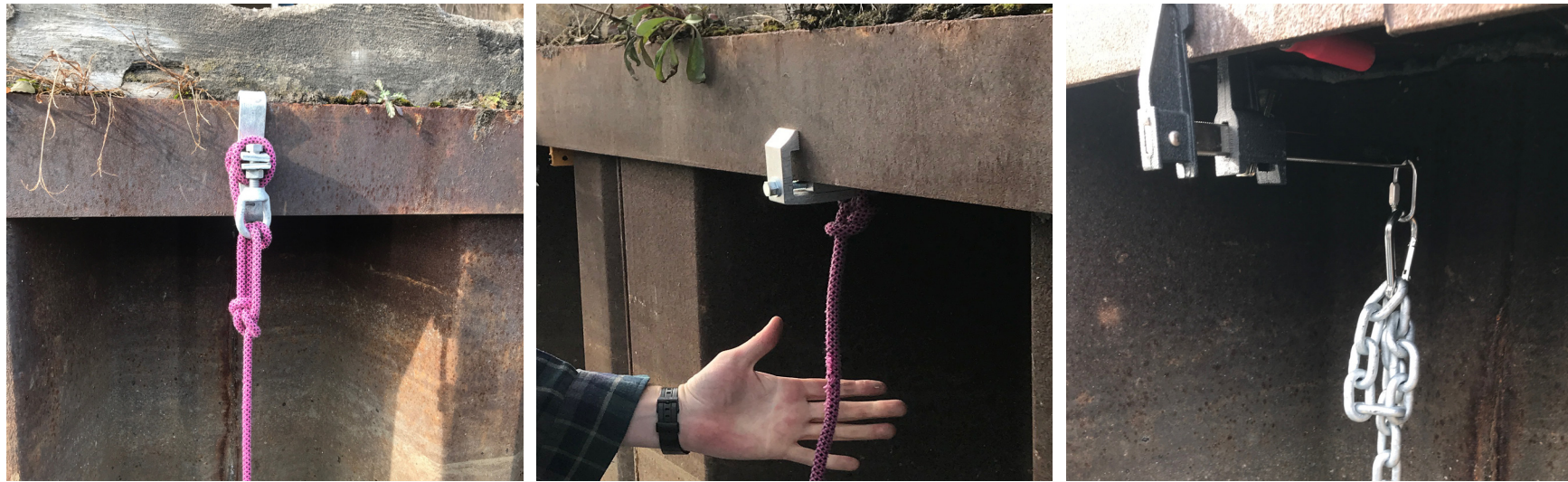
The team tested three different attachment methods, for strength and use of space.
